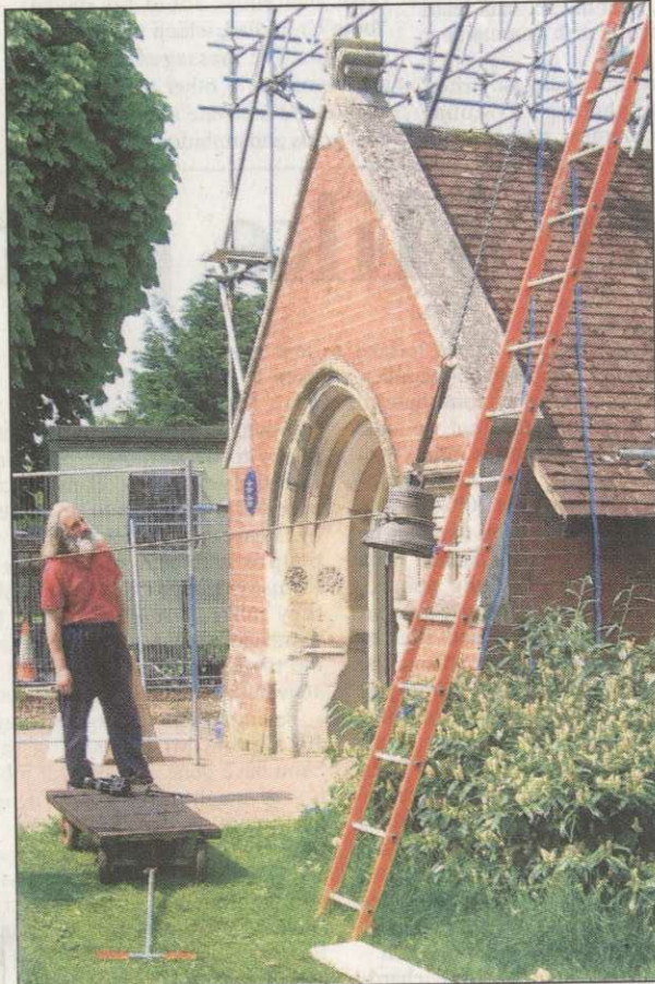
Going up... the new bell being hoisted into the tower of Romsey Library
